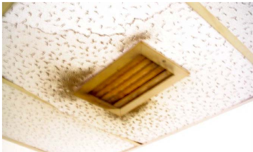
This picture shows mold that is growing around a vent.
